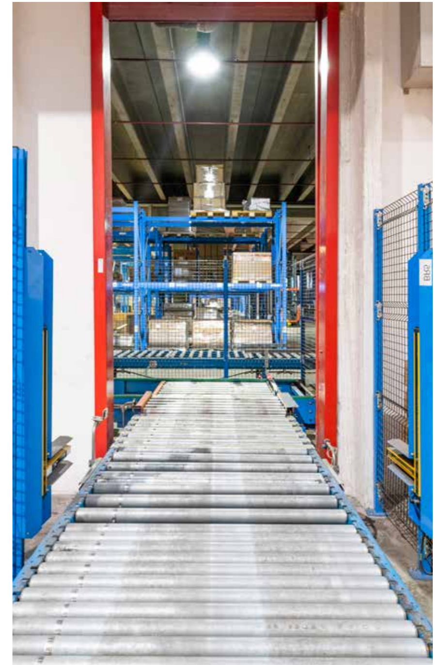
Automatic Shipping Warehouse - Artemide Factory Pregnana Milanese
